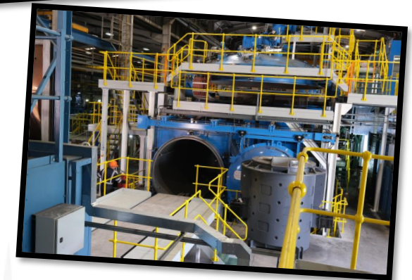
Our latest State-of-the-art furnace installed in 2023
