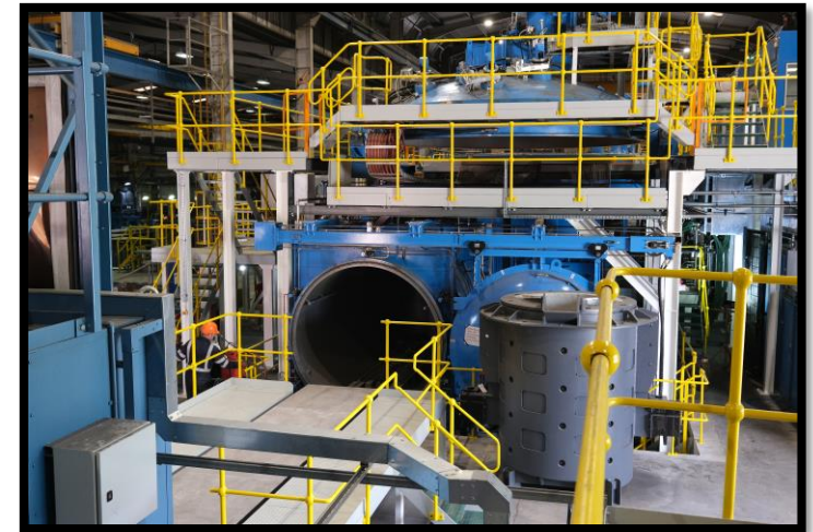
New 4t furnace commissioned June 2023
